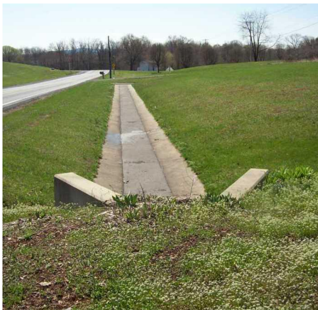
Figure 9. Concrete stormwater conveyance directing runoff downhill toward Elks Run
